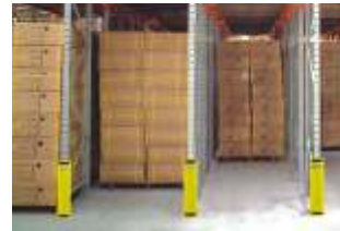
Use an independent steel guard for ends of racks and intersecting gangways
